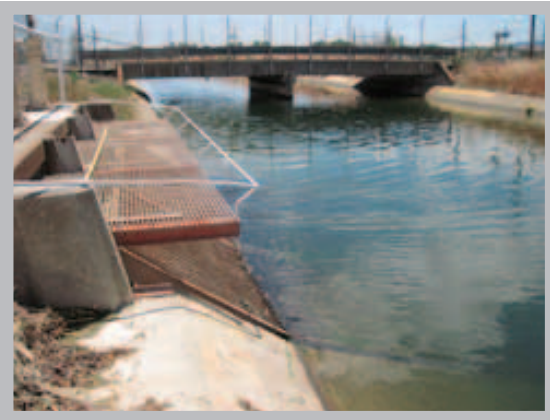
Putah South Canal - Trash rack at Weyand Canal
