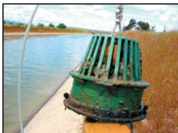
"Putah Trap" after removal from canal
